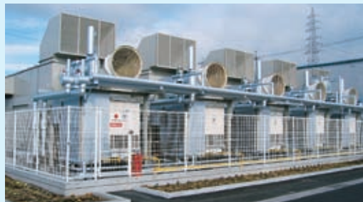
Cogeneration facility of Tobu Factory
