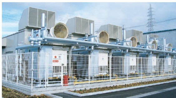
Cogeneration facility of the Tobu Factory
