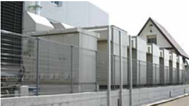
Cogeneration facility at the Naoetsu Plant
