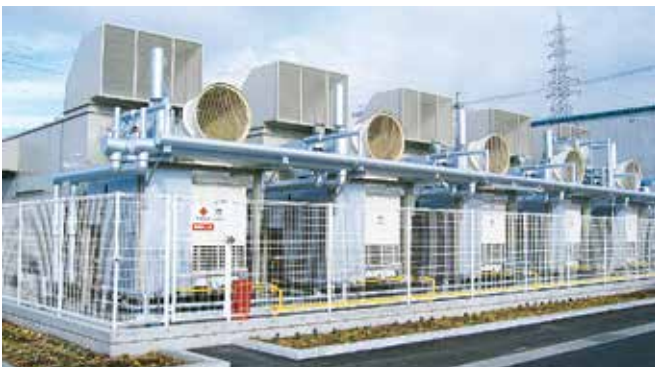
Cogeneration facility at the Tobu Plant
